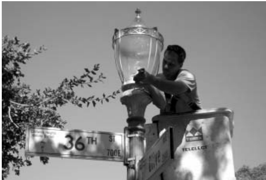
City Light and Power's Chris Fett installs one of 36 restored lamppost tops in Cal Heights.
